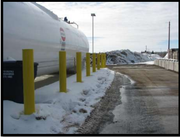
Fuel Station Tank, Bollards, and Lights Looking West
