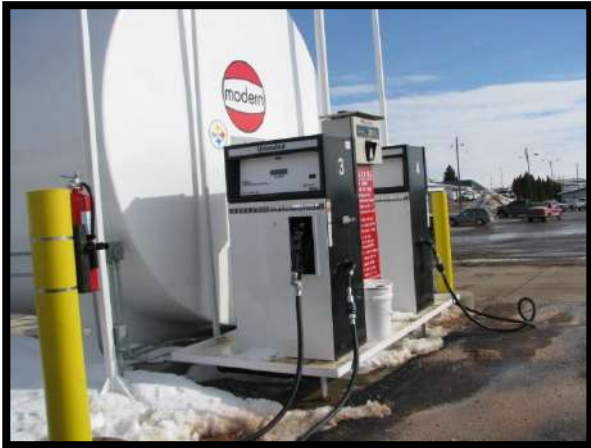
Fuel Station Dispensing
