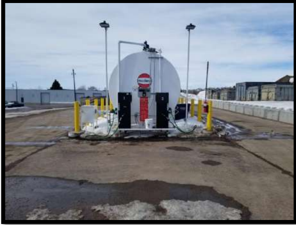
Fuel Station & Dispensers, View Facing West
