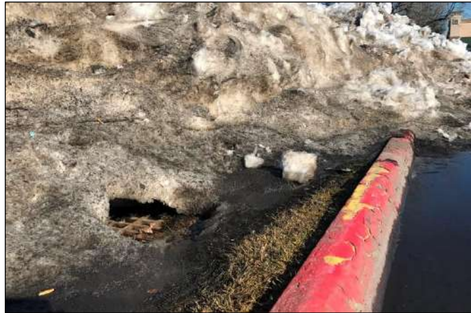
Figure 4-4. Snow on Storm Drain Inlet
