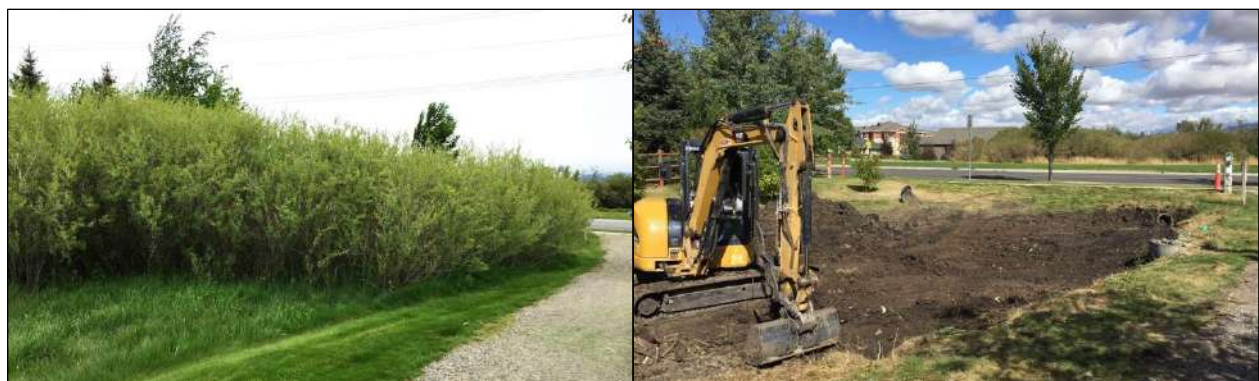
Figure 5.7-6. Detention Basin Deferred Maintenance
