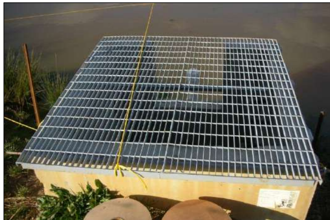
Figure 5.8-5. Outlet Structure Trash Rack
