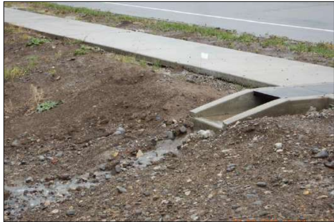
Figure 5.6-6. Degrading Concentrated Flow Inlet Source: HDR
