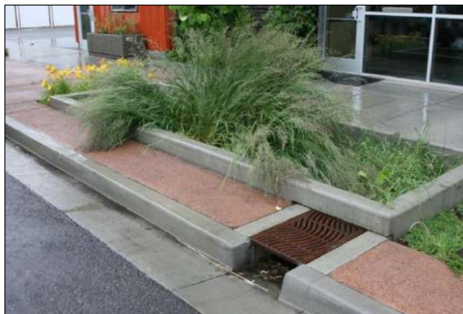
Figure 5.3-6. Offline Bioretention Area
