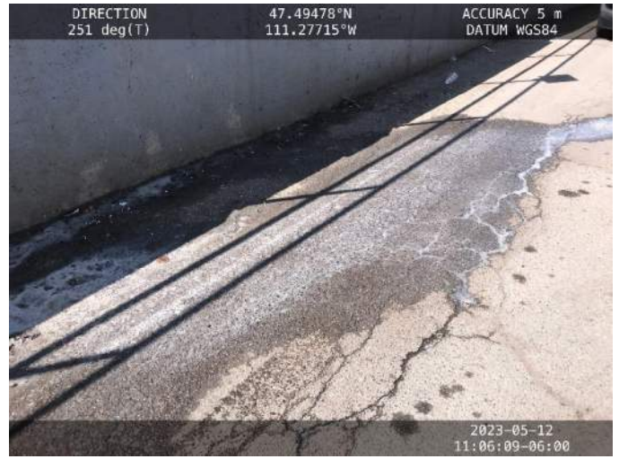
Observed coloration in discharge (5/12/23)
