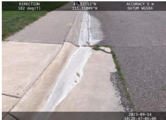
3. Concrete washout flowing along curb line downhill.
