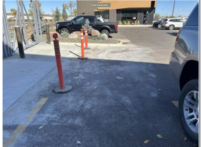
Photo shows general extent of the issue surrounding the trash enclosure
