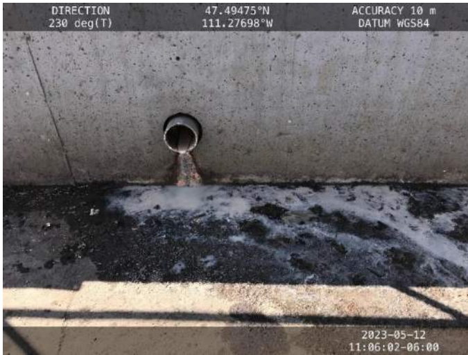
Observed coloration in discharge (5/12/23)
