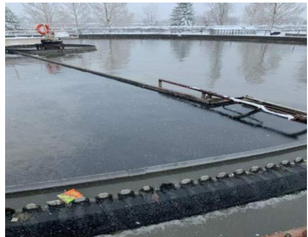
4. Oil in treatment pond
