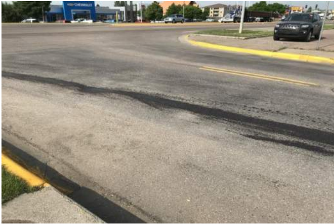
Oil stain can be seen on roadway coming off 10 th Ave So and 40 th St So.
