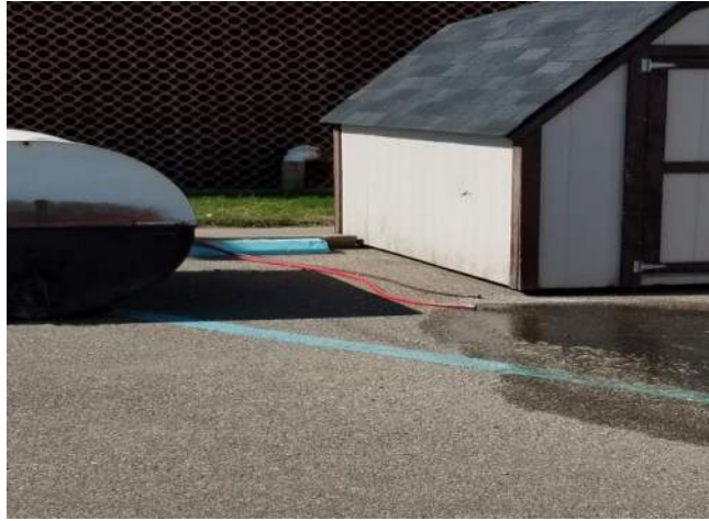
1. Water being pumped from building into parking lot with garden hose.
