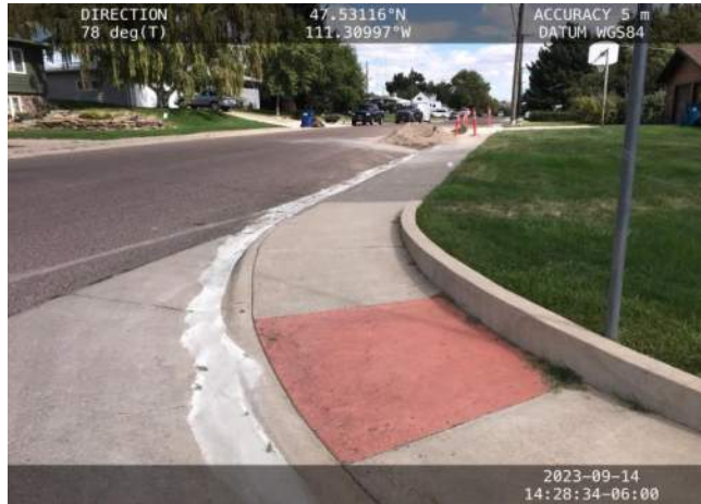
1. Concrete washout flowing along curb line from stockpile at 156 Riverview 3E.
