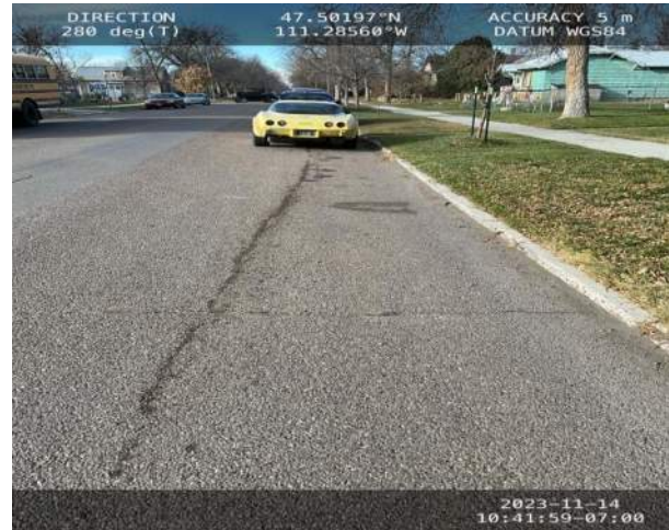
Oil stains were seen in front of other residences as well.
