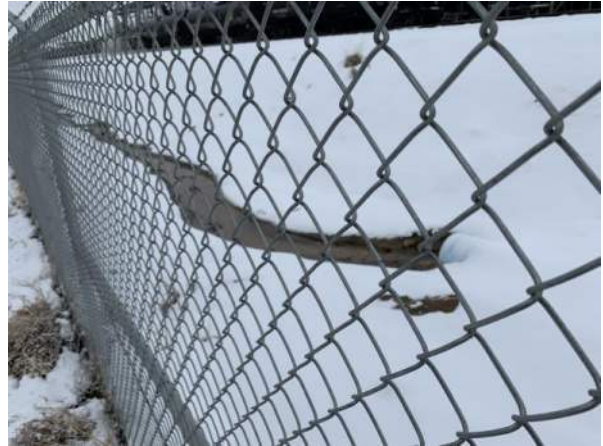
2. Oil sheen flowing into culvert along tracts.
