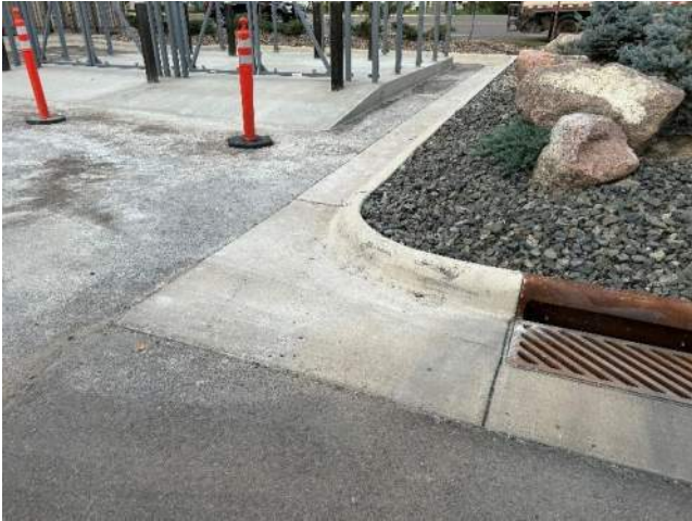
Photo shows concrete washout/cement material from dried ramp work traveling down to the storm inlet
