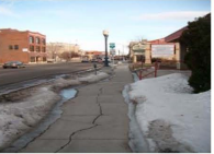
Poor Street & Sidewalk Maintenance
