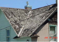
Deteriorating Residential Buildings
