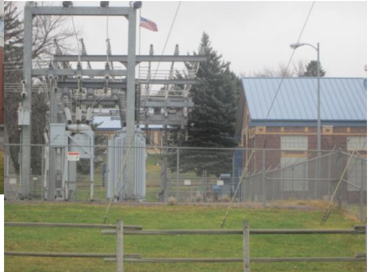
LOCATION OF EXISTING SUBSTATION, SHOWING DESIGN OF THE PUMP STATION (FOREGROUND), FILTER BUILDING (BACKGROUND).
