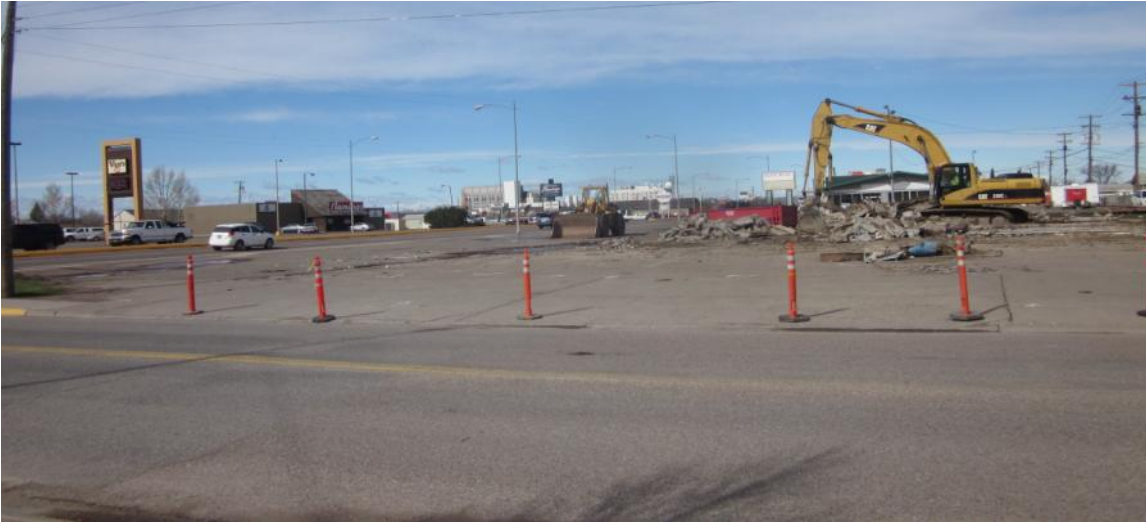
View west from 32nd Street South at demolition of the gas station on the subject property.
