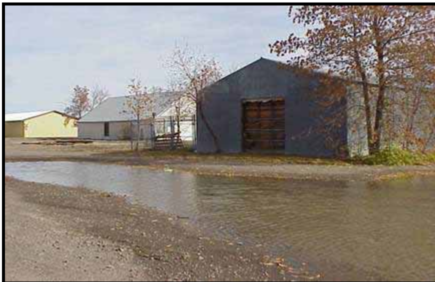
Figure 9. Drainage Problems South of 1st Avenue Southwest, Looking North
