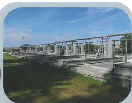
The coagulation and flocculation process occurs at this location in underground chambers.
