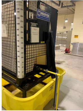
The line was originally plumbed directly down and the tote had to be filled from the top.
