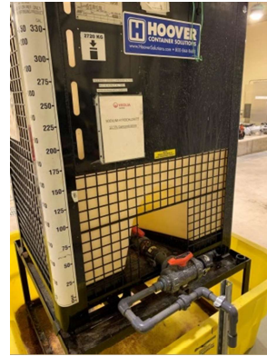
The line was re-plumbed to allow filling of the tote from ground level.
