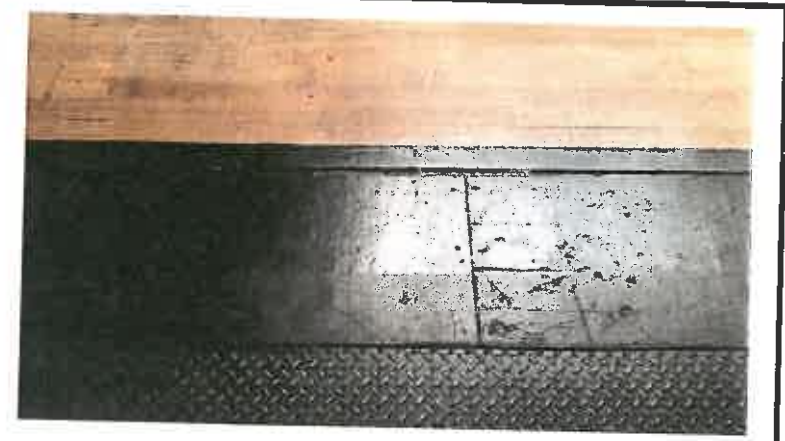
Replace black painted wood area with a steel plate that is shored up from below.
