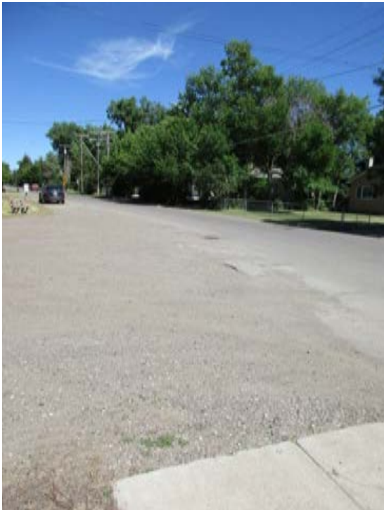
2. Looking east along 10 th Avenue Southwest sidewalk end and gravel extends to public ROW
