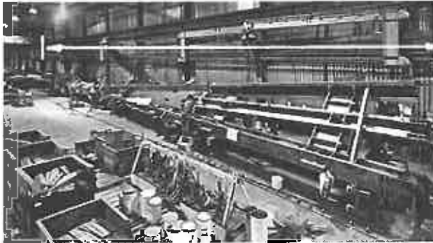
One of the corner nodes near the 20th floor (New York, NY, U.S.A.)
