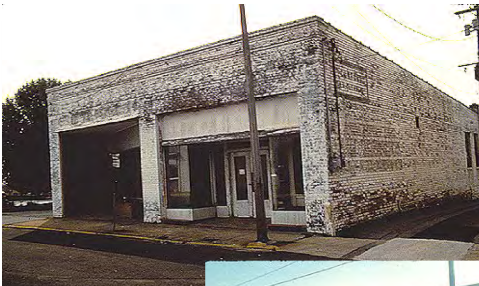
An example of rehabilitation of a dilapidated building, using simple architectural design solutions and structural improvements.
