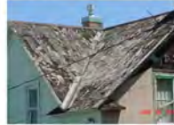
Deteriorating Residential Buildings
