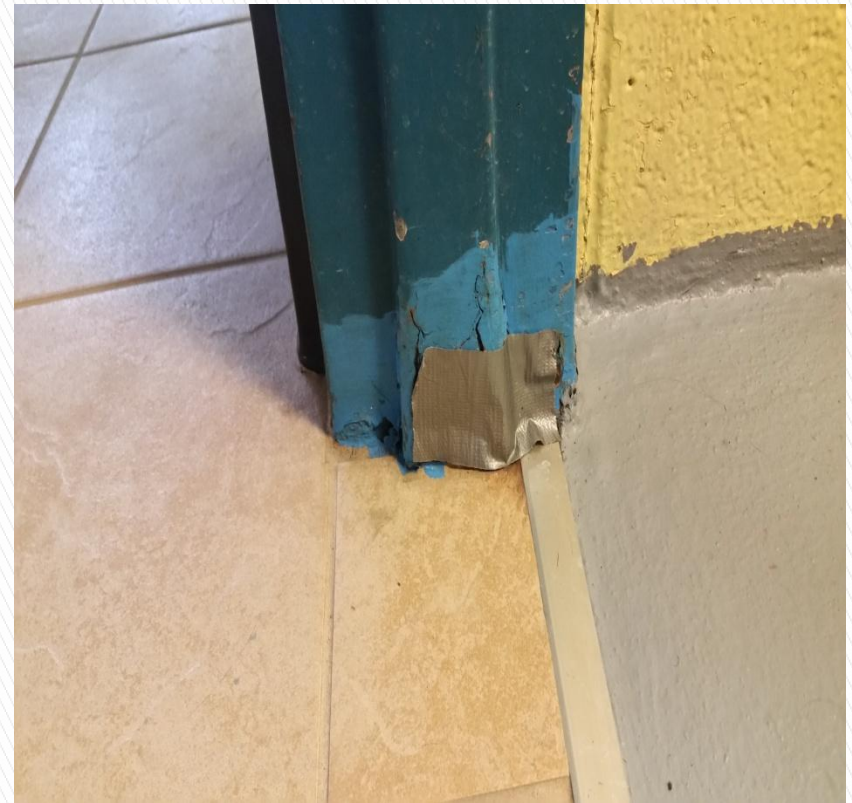
Rusted Interior Doors
