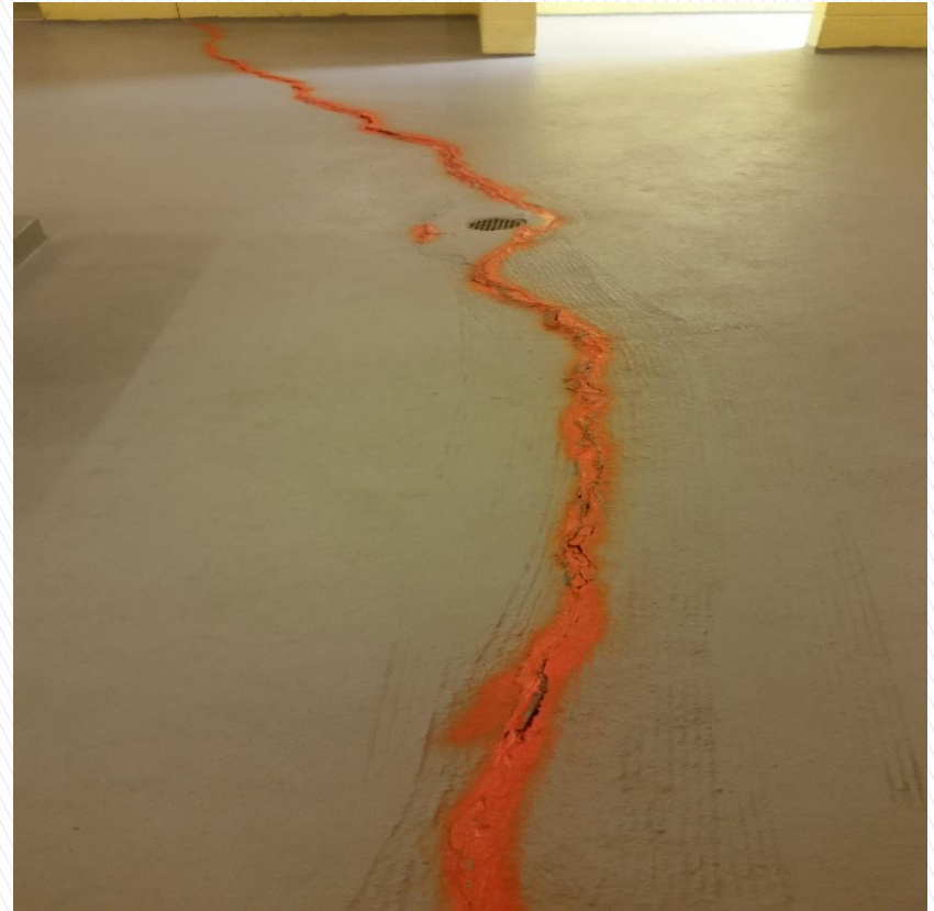
Women's Locker Room Floor Crack (sinking)
