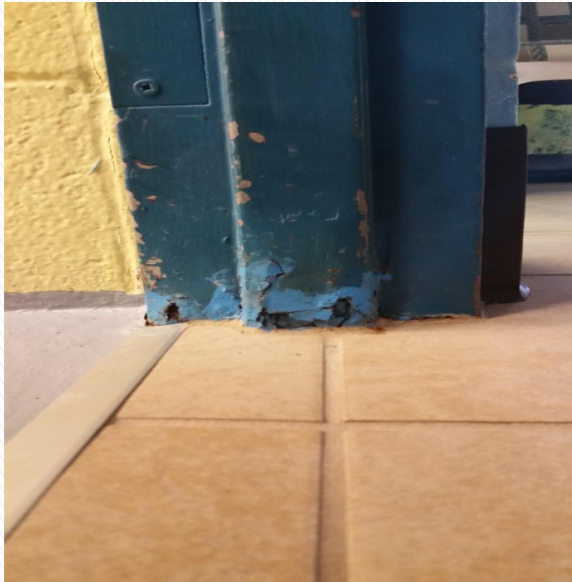
Rusted Interior Doors
