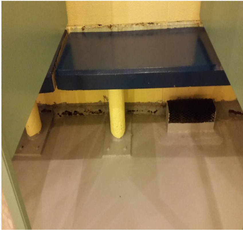
Wall Separation Women's Room
