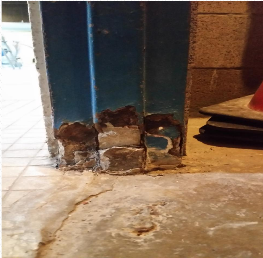
Rusted Interior Doors
