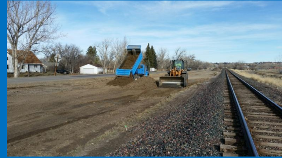
An estimated 35,000 cubic yards of fill material was used to improve drainage and safety on shoulders of Lower River Road.
