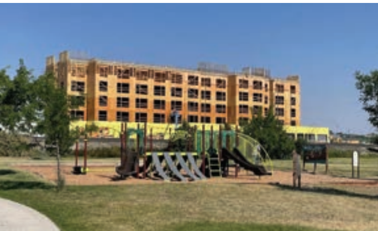
The TownePlace Suites under construction in West Bank Landing will add over 100 extended stay hotel rooms to grow our tourism industry.
