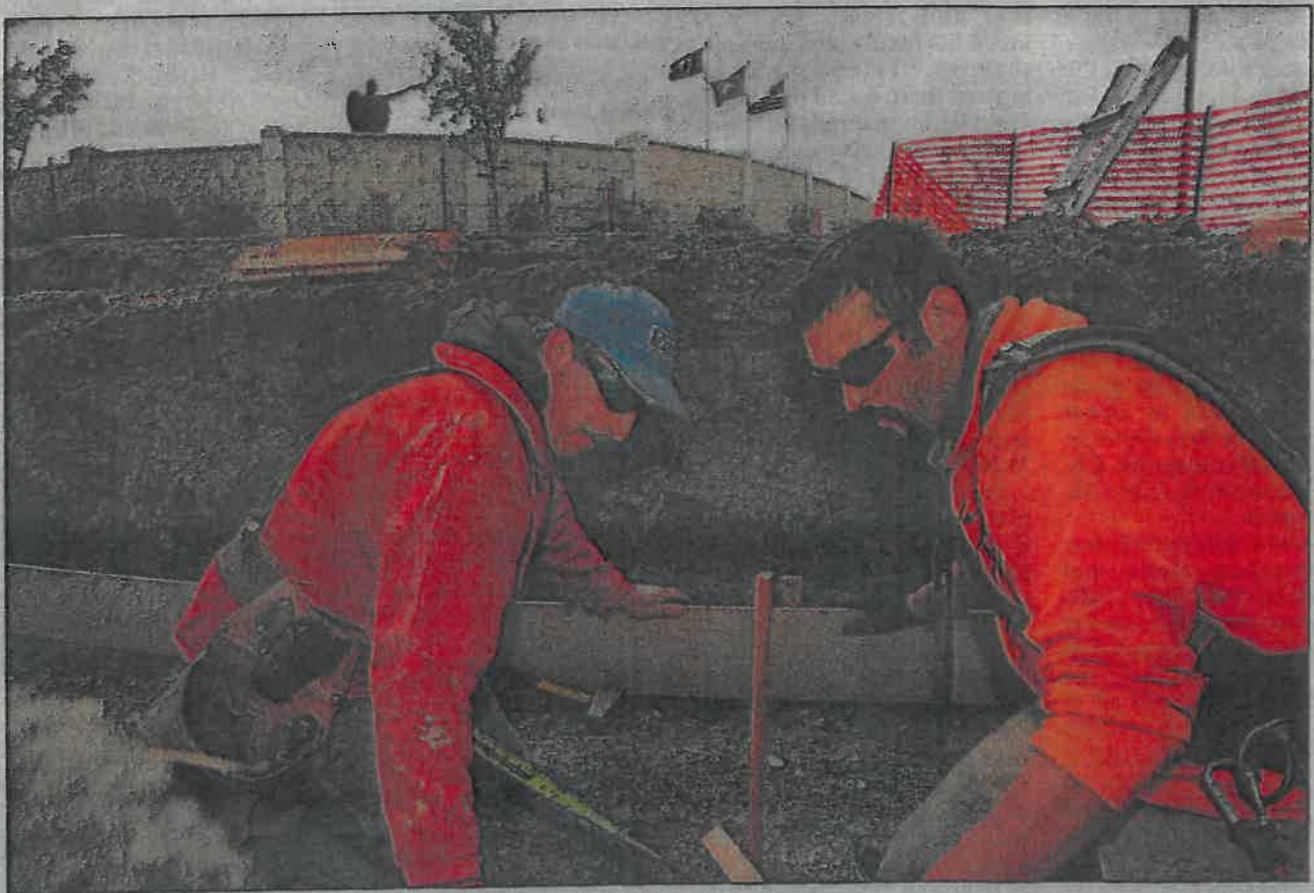
Ken Reiner, left, and Seth Phelps of Dick Olson Construction set up forms as an expansion project begins at the Montana Veterans' Memorial on Wednesday afternoon. TRIBUNE PHOTO/ION SANDERS
