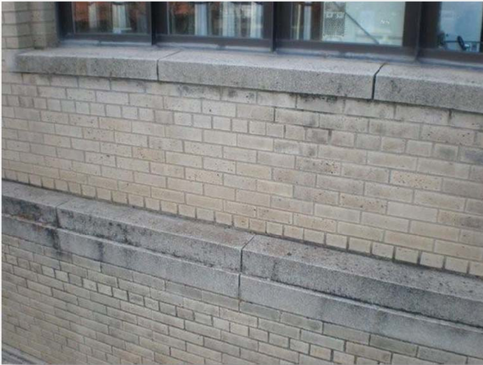
Photo N5 – Typical Weathered Mortar Joints
