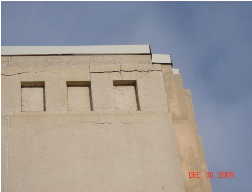
Figure 1. View of cracking on upper part of Civic Center (NTL).
