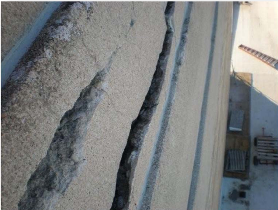
Photo W8 – Large Open Cast Panel Cracks
