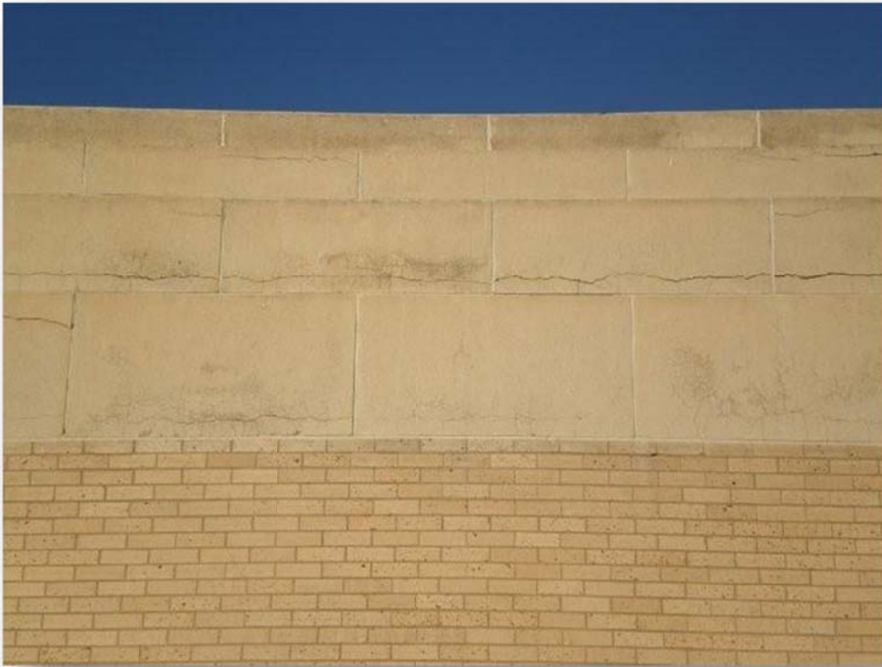
Photo W7 – Typical Cracking Cast Panels
