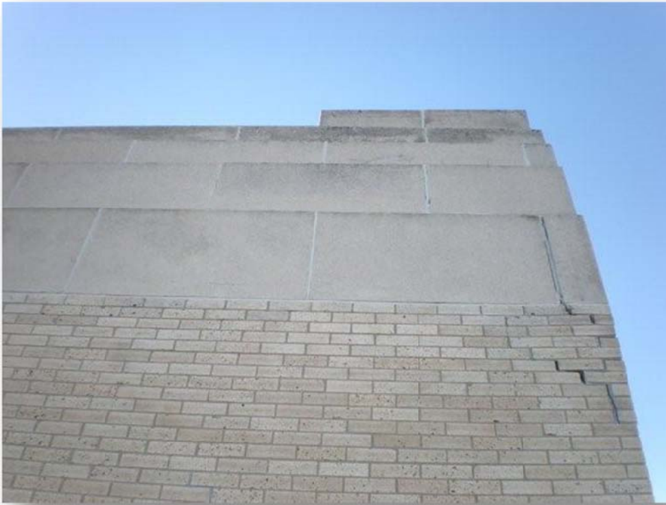
Photo N1 – Typical Cracking Cast Panels & Displaced Brick
