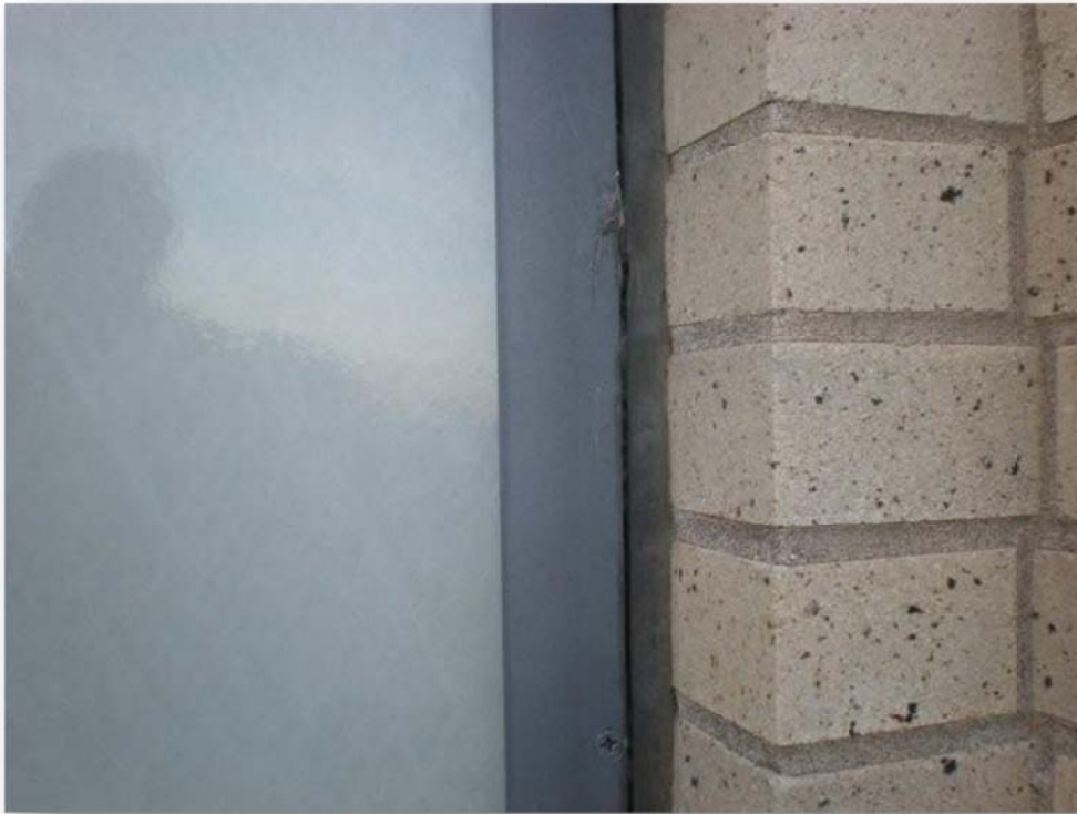
Photo W3 – Typical Window Weathered Caulking Joint
