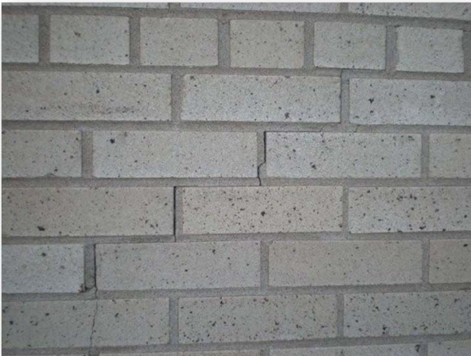
Photo W6 – Brick Cracking
