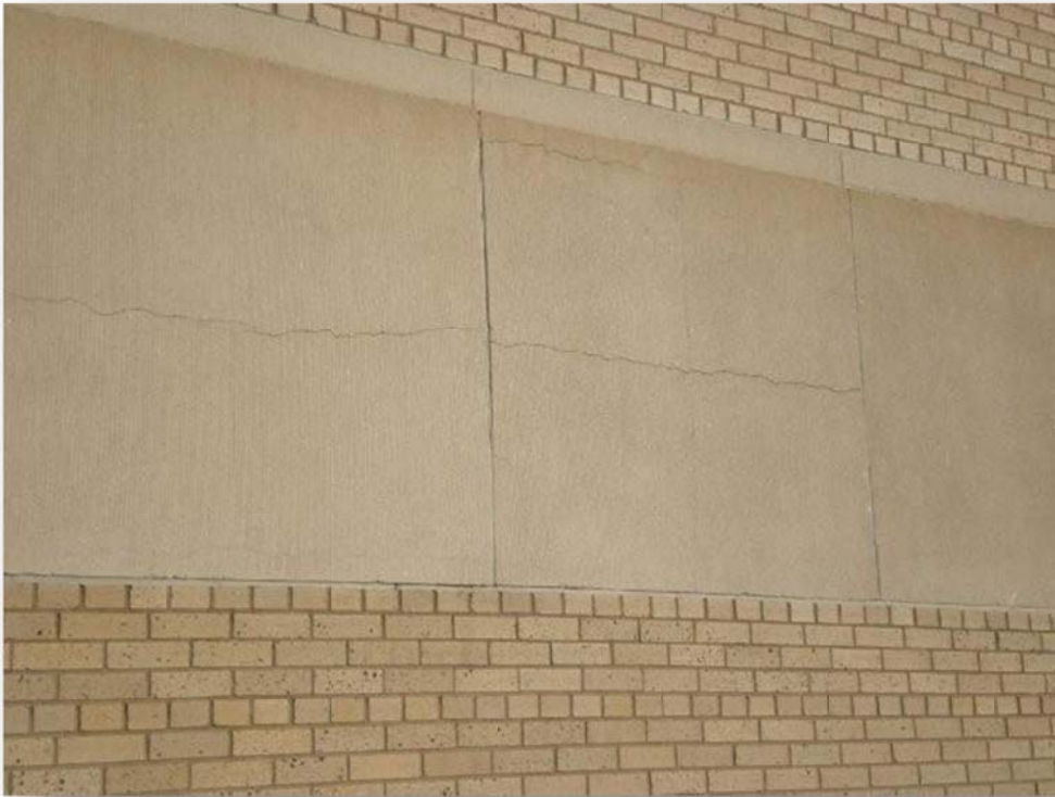
Photo S7 – Typical Cracking Cast Panels
