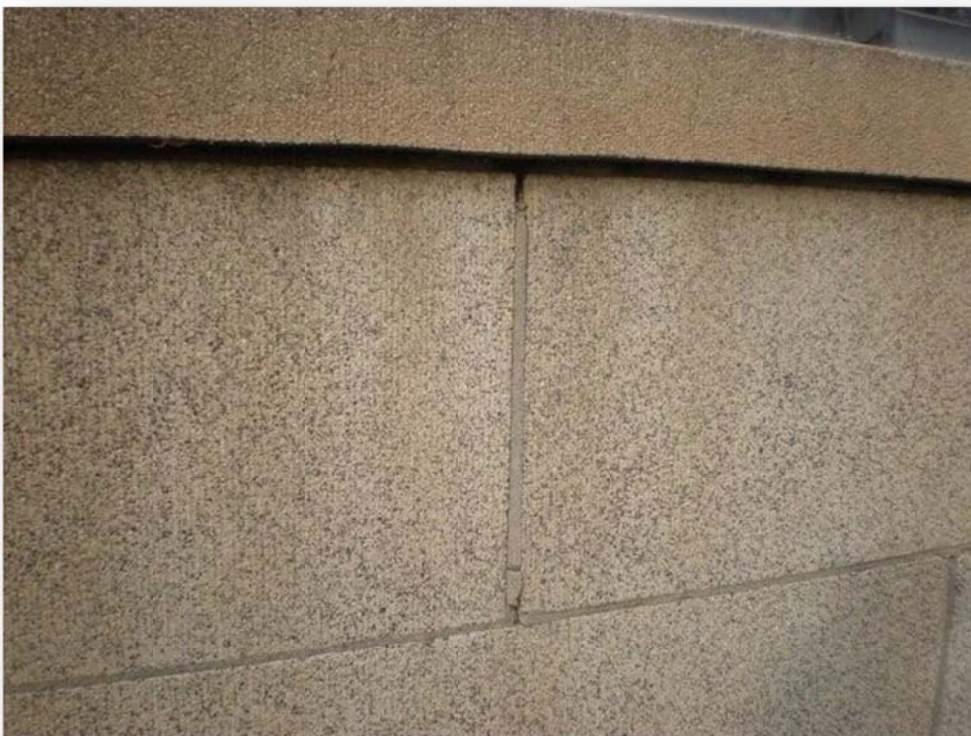
Photo E2 – Typical Weathered Mortar Joint
