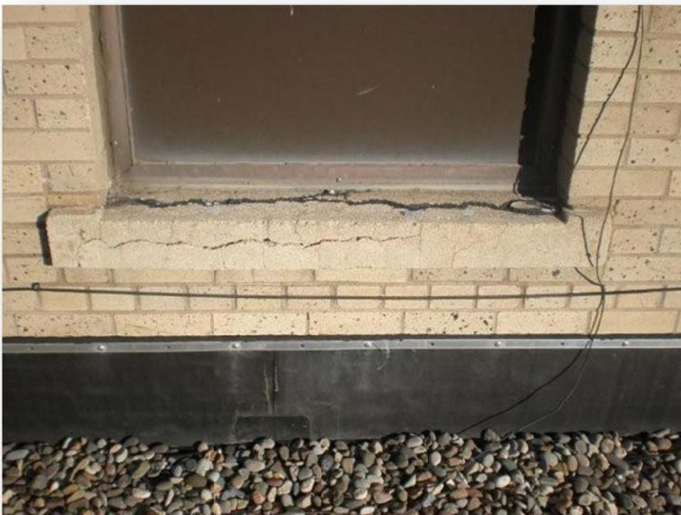
Photo S6 – Cracked Cast Window Sill
