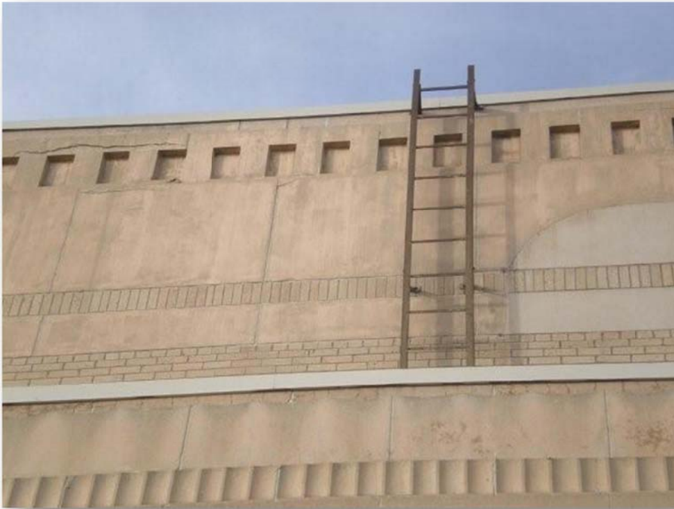
Photo E5 – Typical Cracking Cast Panels
