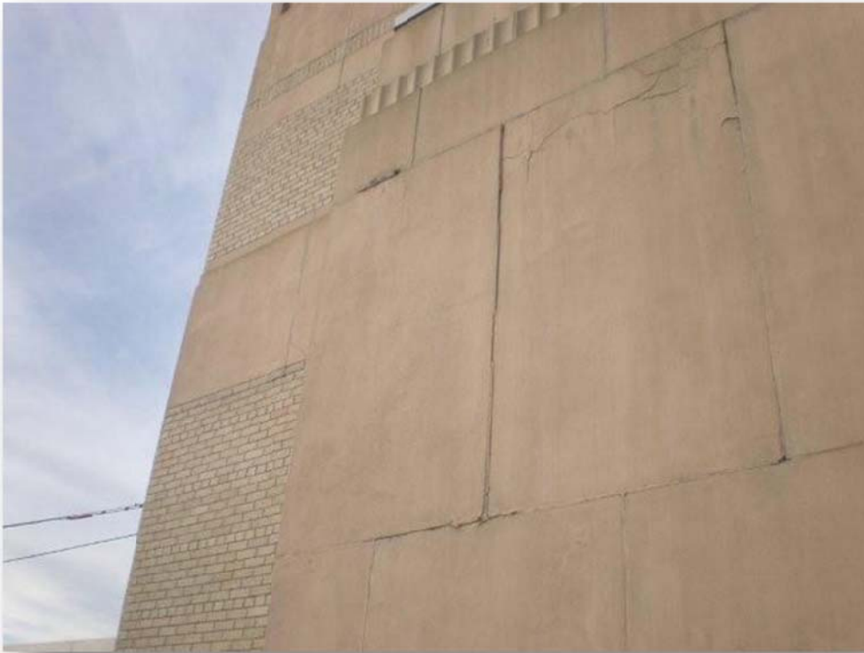
Photo E3 – Typical Cracking Cast Panels
