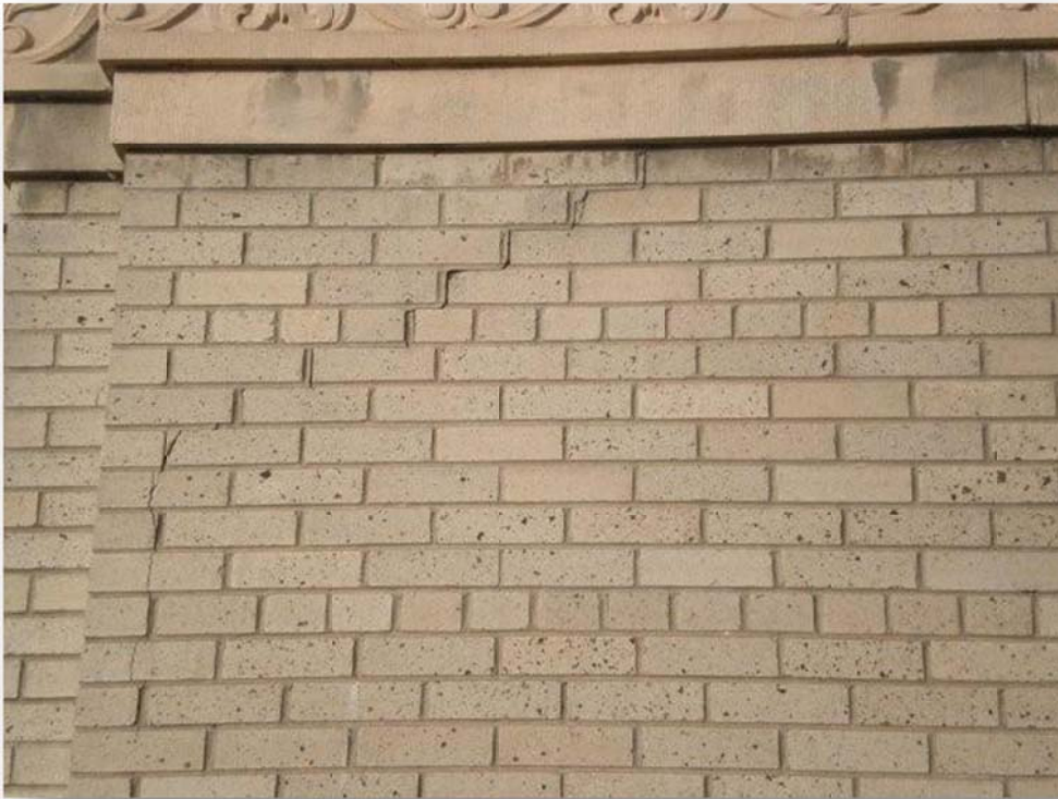
Photo E1 – Cracked and Displaced Brick
