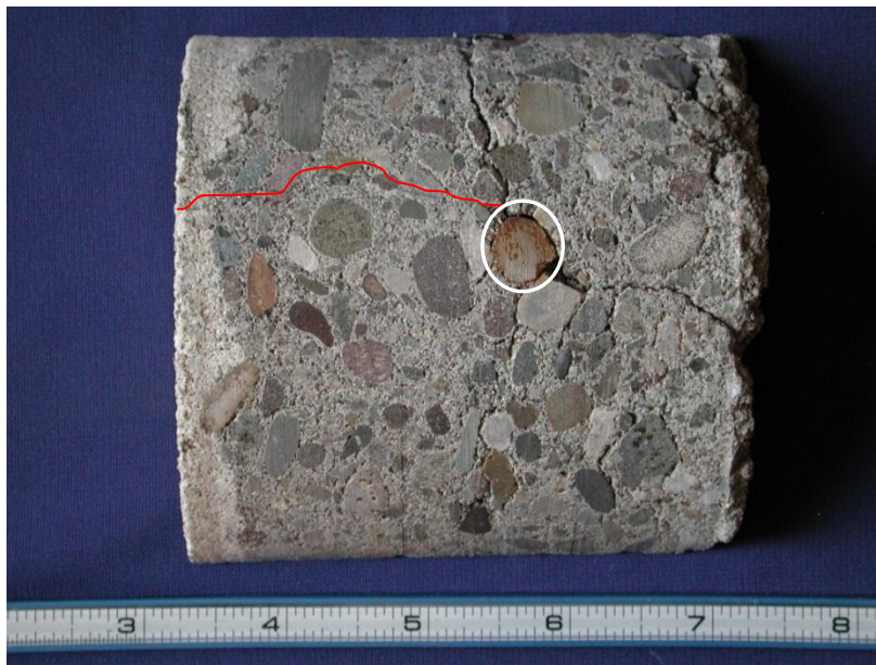
Figure 4. Side view of the core. Cracks radiate from the corroded reinforcing bar. One fine crack to the surface is outlined in red. The irregular cracks in the photo located to the right of the (encircled) rebar and oriented parallel to the inner surface coincide with abundant air voids that are typical of dry cast concrete.
