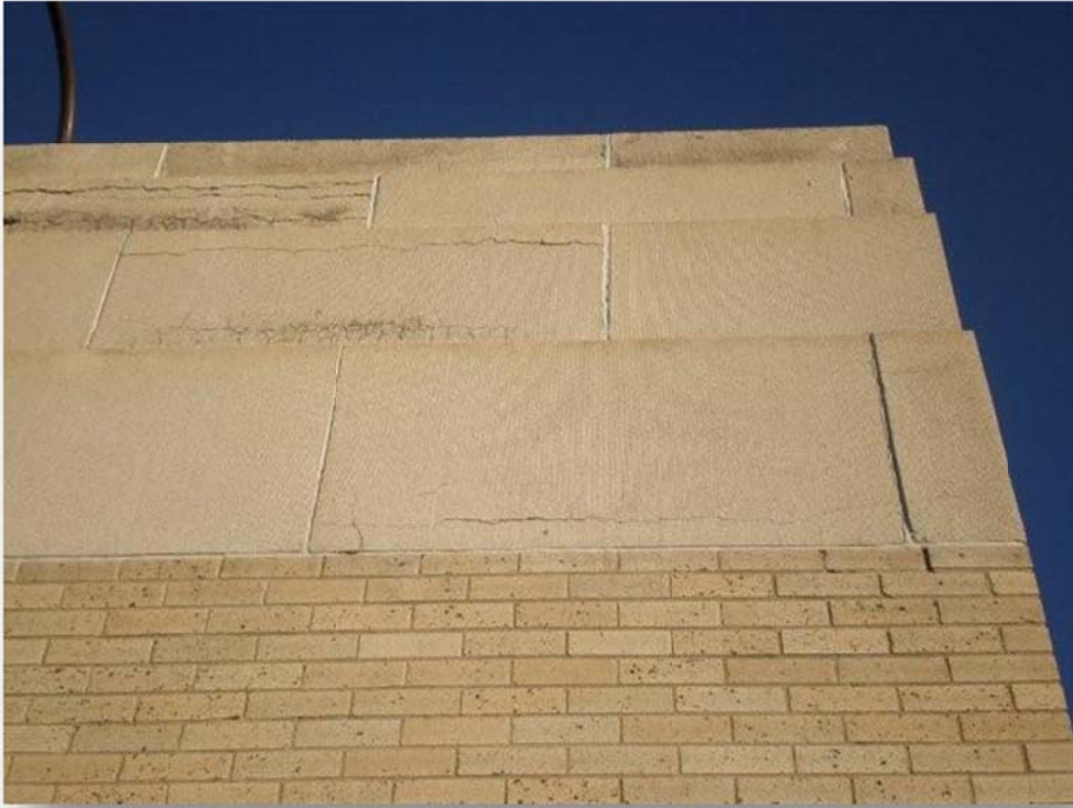
Photo S1 – Typical Cracking Cast Panels
