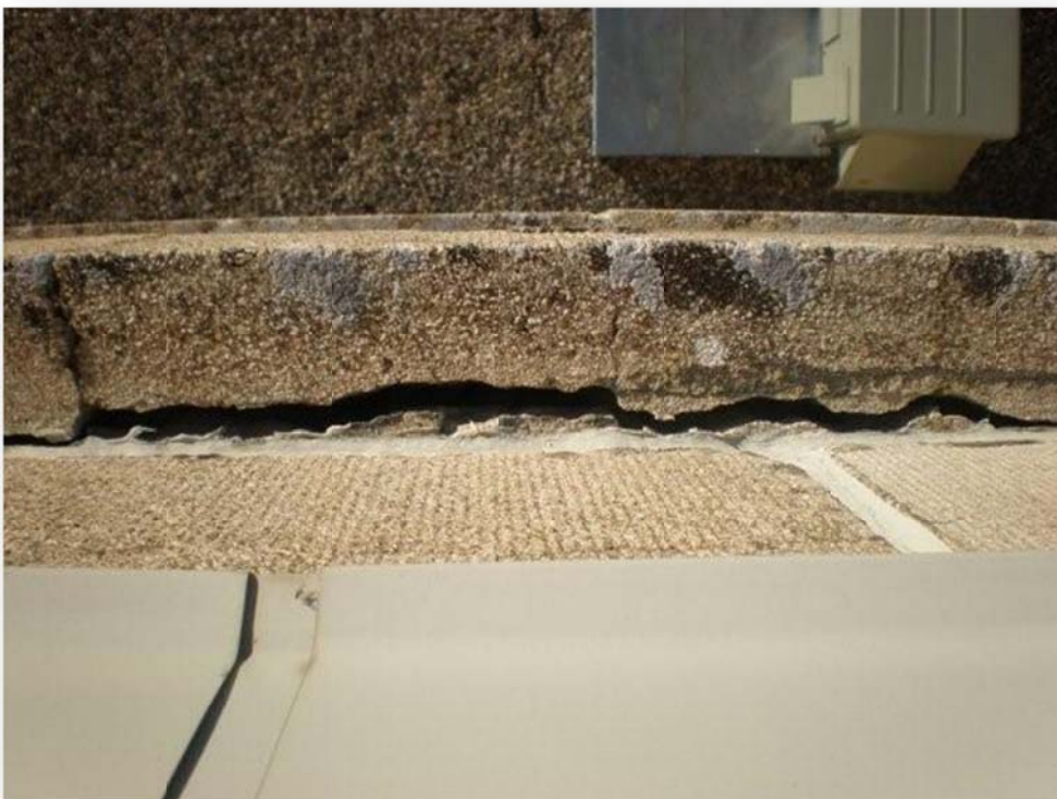
Photo S4 – Large Open Cast Panel Cracks
