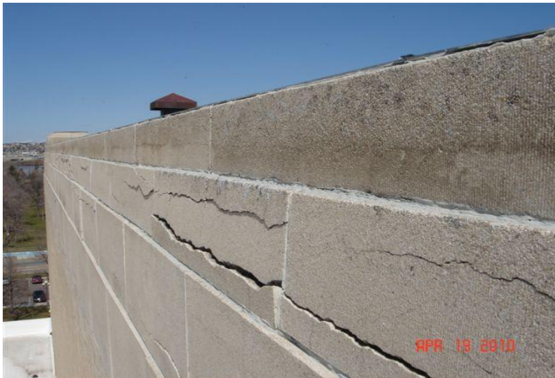
Figure 2. View of cracking caused by corrosion of embedded reinforcing steel (NTL).
