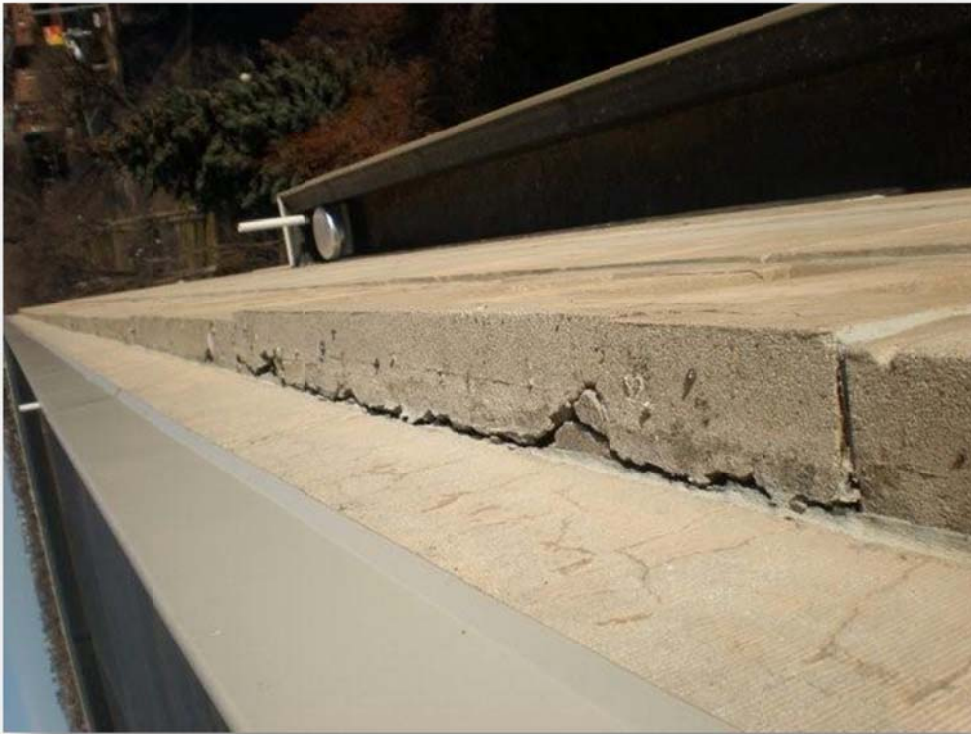
Photo E7 – Typical Cracking Cast Panels
