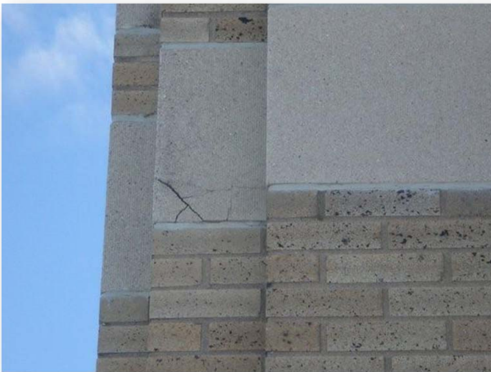
Photo N2 – Typical Cracking Cast Panels
