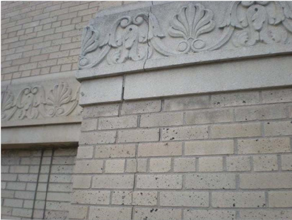
Photo N7 – Typical Cracking Brick & Weathered Mortar Joints
