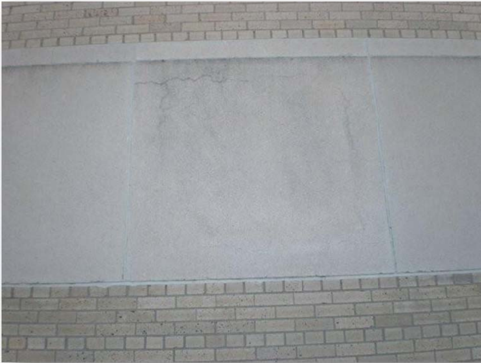
Photo N3 – Typical Cracking Cast Panels
