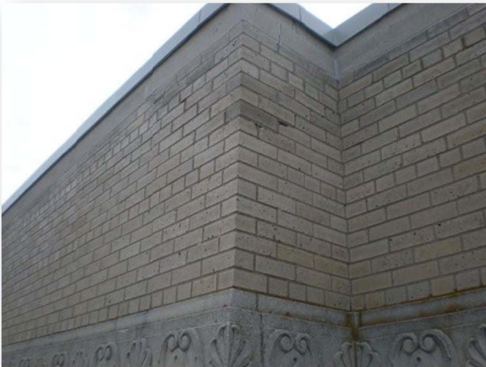
Photo N6 – Typical Weathered Mortar Joints & Displaced Brick
