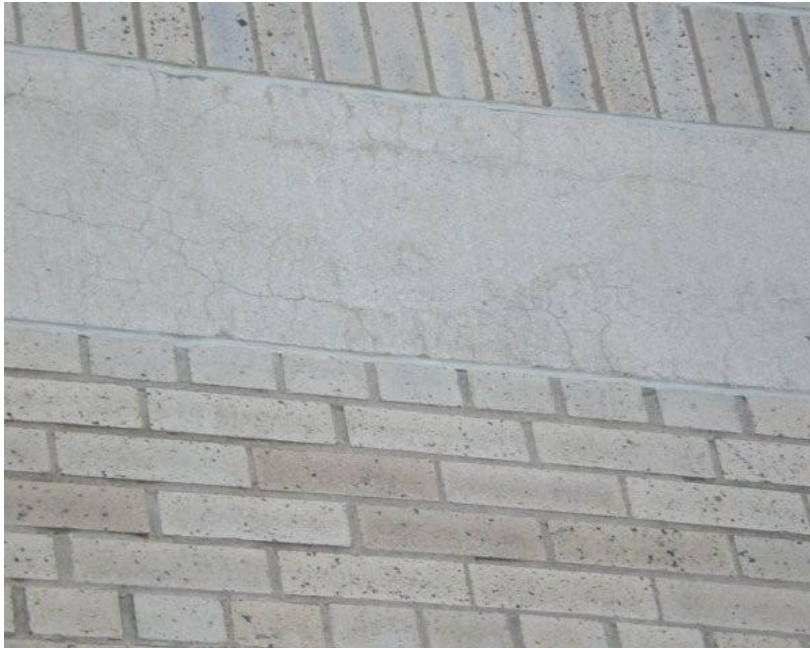
Figure 3. View of the fine cracks on panels that are currently in good condition (NTL).
