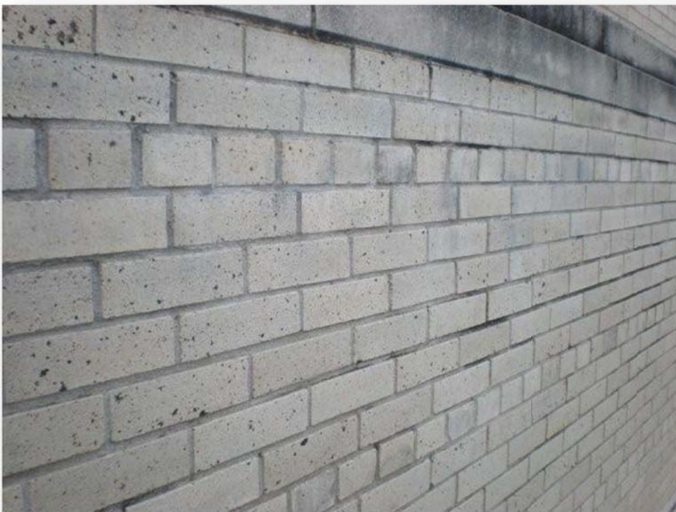
Photo N8 – Typical Weathered Mortar Joints
