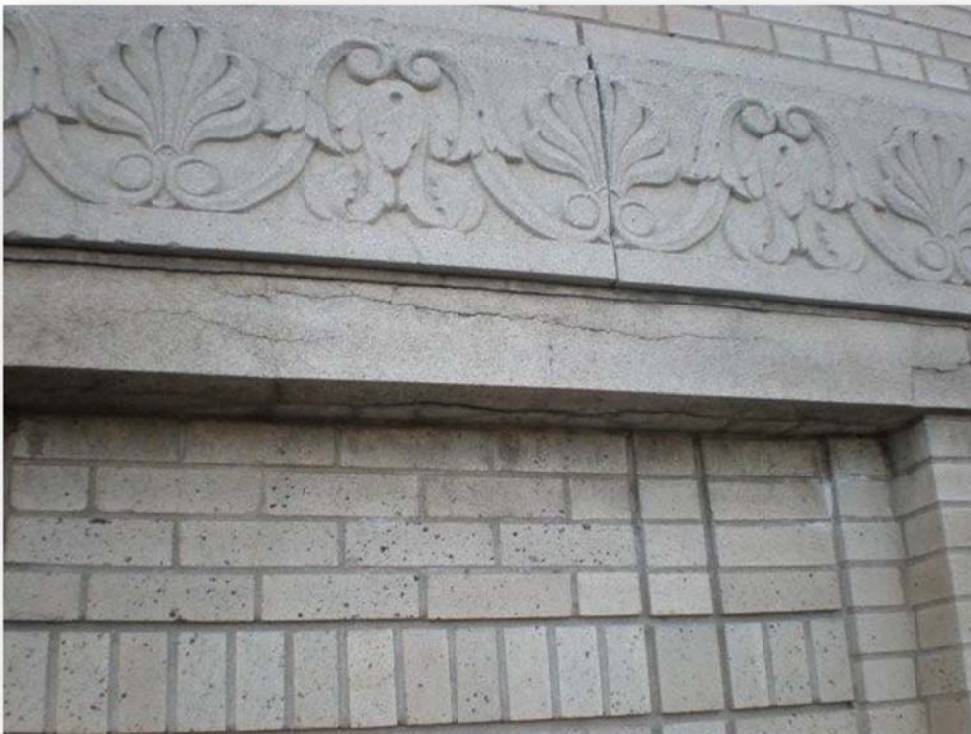
Photo W2 – Typical Cracked Lintel Block
