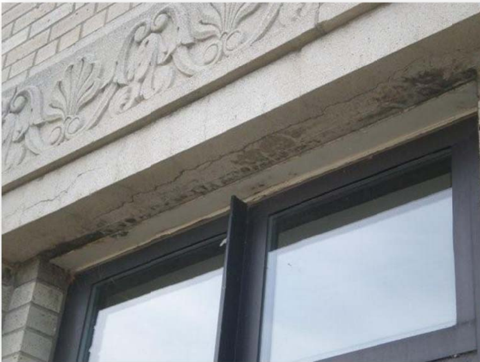
Photo N4 – Typical Cracked Window Lintel
