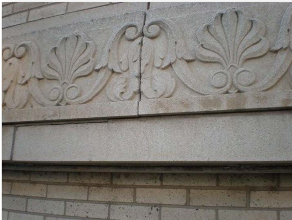
Photo W4 – Typical Weathered Mortar Joints
