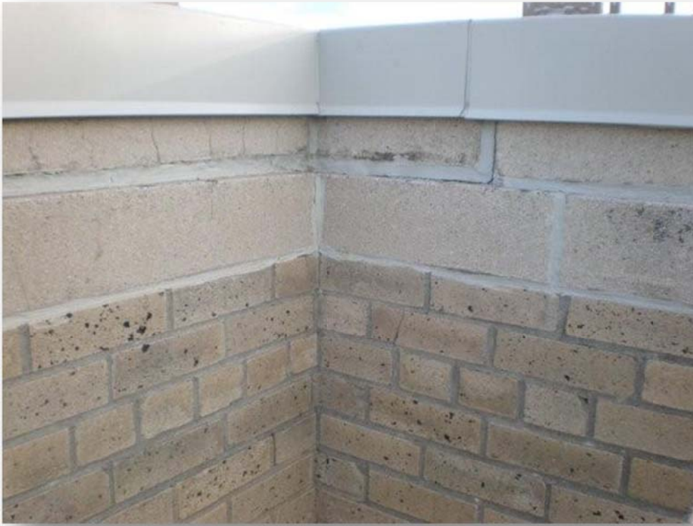
Photo S11 – Typical Cracking Cast Panels at Parapet Level
