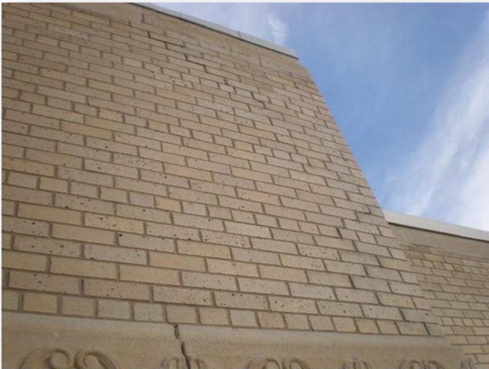
Photo S10 – Cracked & Displaced Brick
