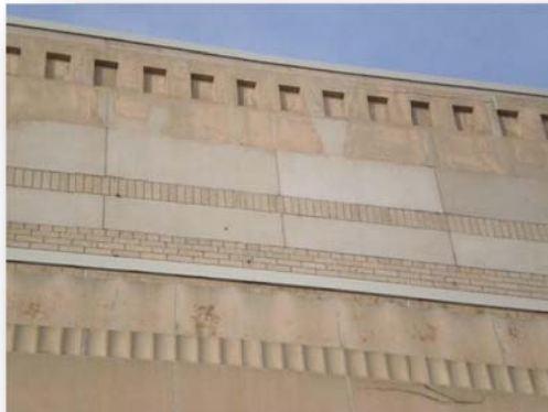
Cast Panels with Pinkish Tint Highlighted by the Area Where the Marquee Sign Was Removed
