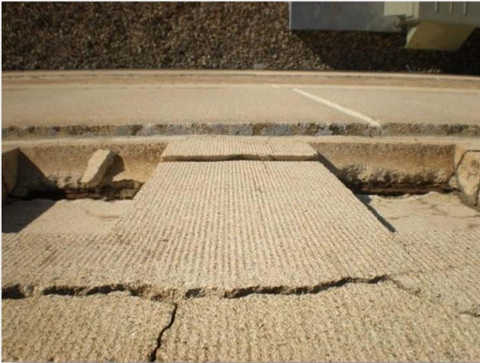
Photo S5 – Typical Cracking Cast Panels
