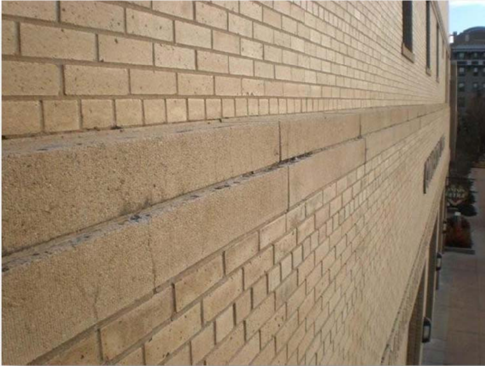
Photo S9 – Typical Cracking Cast Panels
