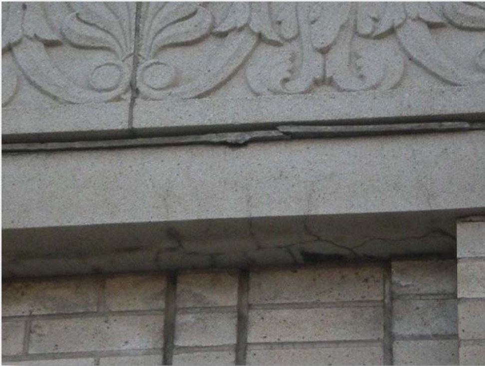
Photo W5 – Typical Cracked Lintel and Weathered Mortar Joints
