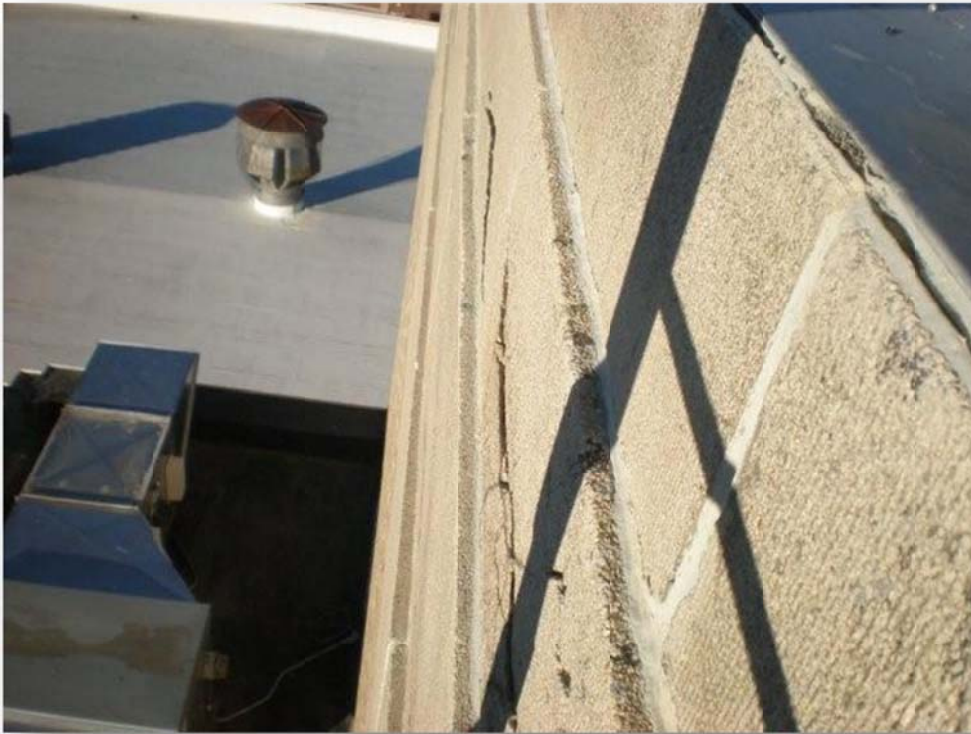
Photo S3 – Typical Cracking Cast Panels
