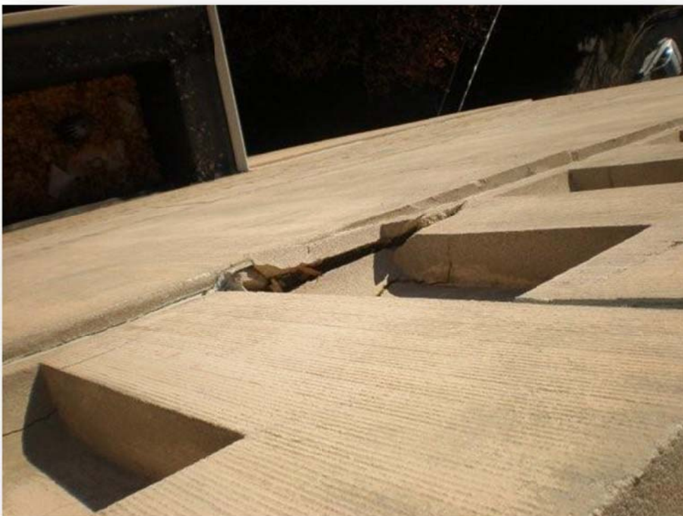
Photo E6 – Typical Cracking Cast Panels
