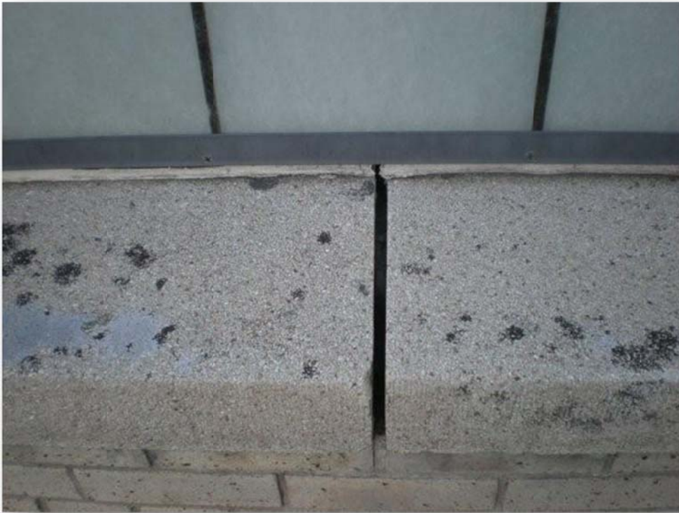
Photo W1 – Typical Window Sill Weathered Mortar Joint
