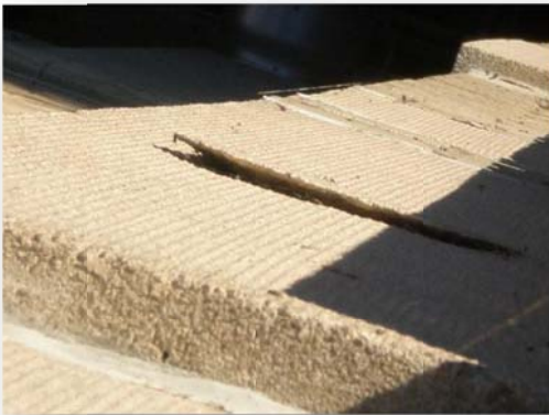
Spalling Panel Face
