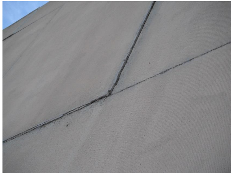
Figure 4 - Noticeable Buckling is Observed on Some Panels
