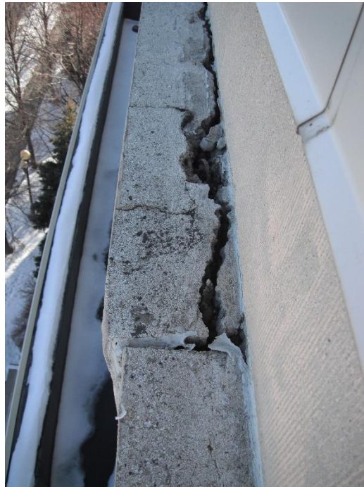
Figure 6 - Major Cracking at Top Edge of Veneer
