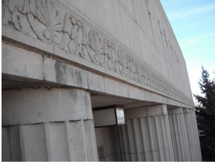
Figure 5 - Some features, such as this frieze, are still in good condition.
